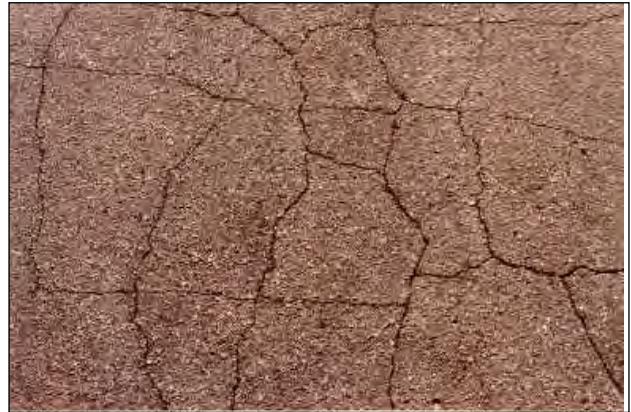
Condition 5 – Very Poor
